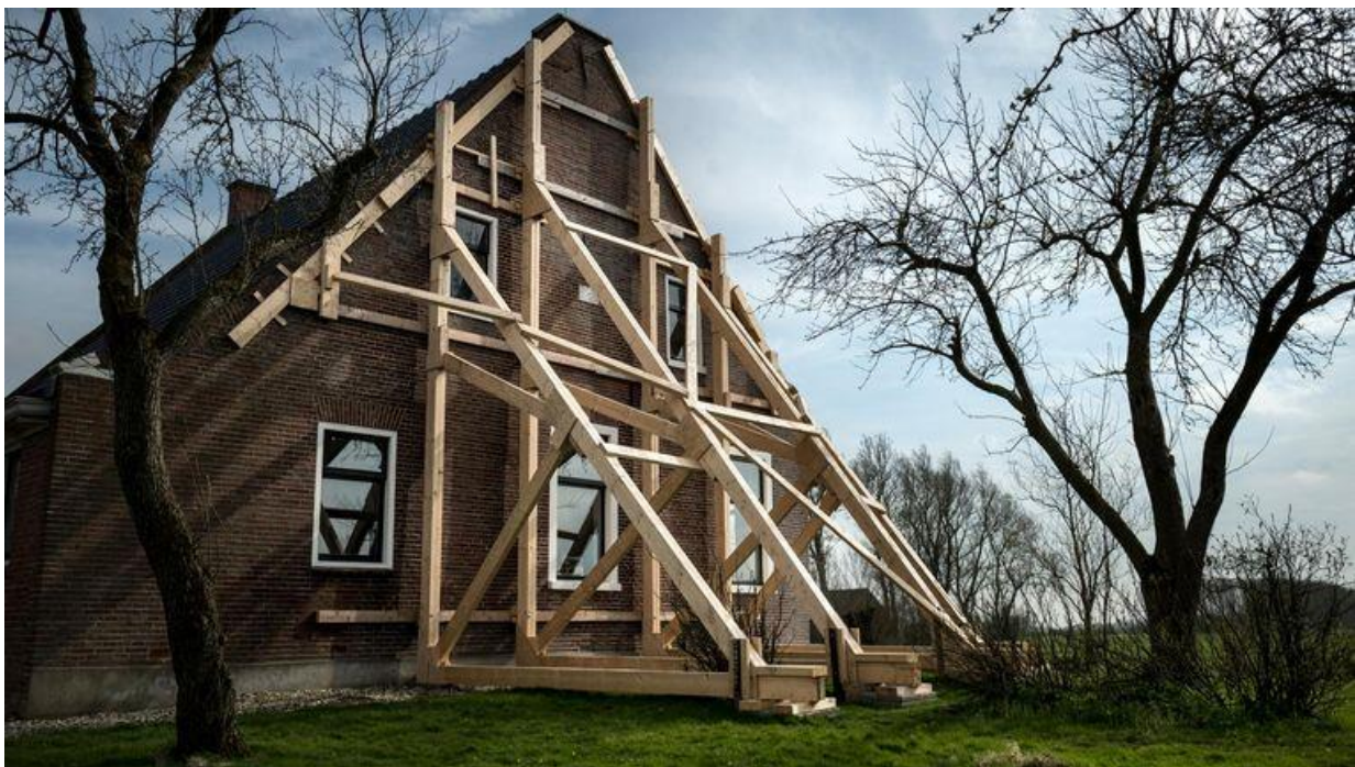
Figure 4: A shored-up house in Groningen. 29
